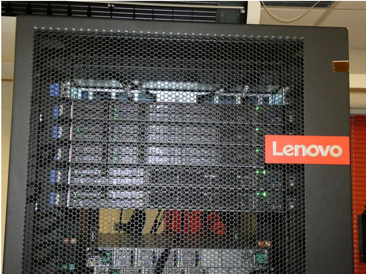
Racks which form part of Northumbria University's new Higgs HPC cluster.
