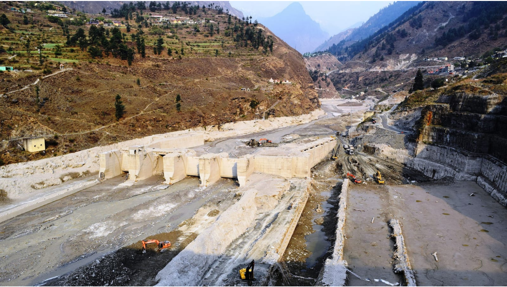
Destroyed Tapovan Vishnugad hydroelectric plant after devastating debris flow of Feb 7, 2021. Photo: Irfan Rashid, Department of Geoinformatics, University of Kashmir.
