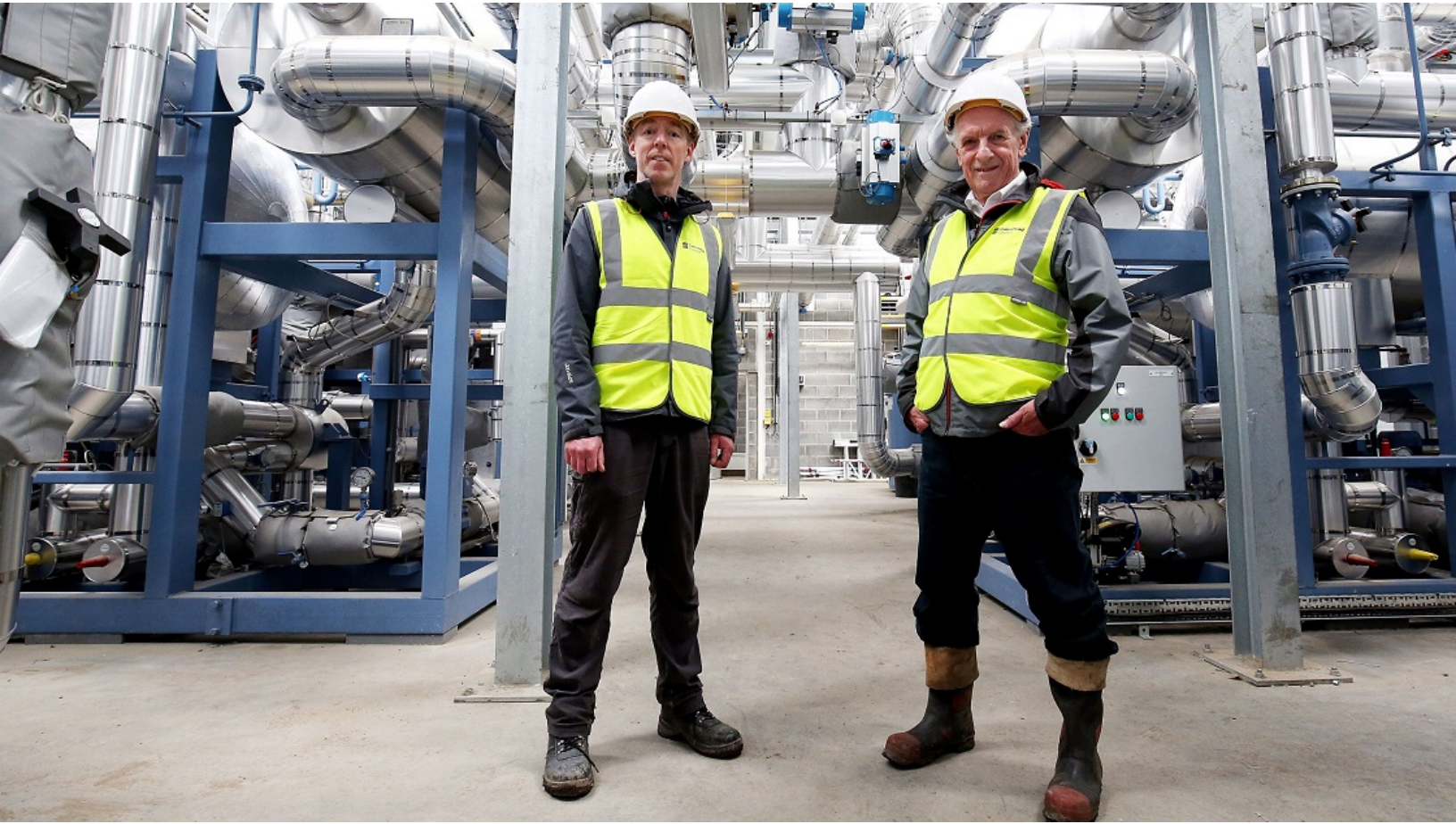
Jim Gillon, Energy Services Manager, Gateshead Council, with Cllr John McElroy, at Gateshead's Energy Centre.
